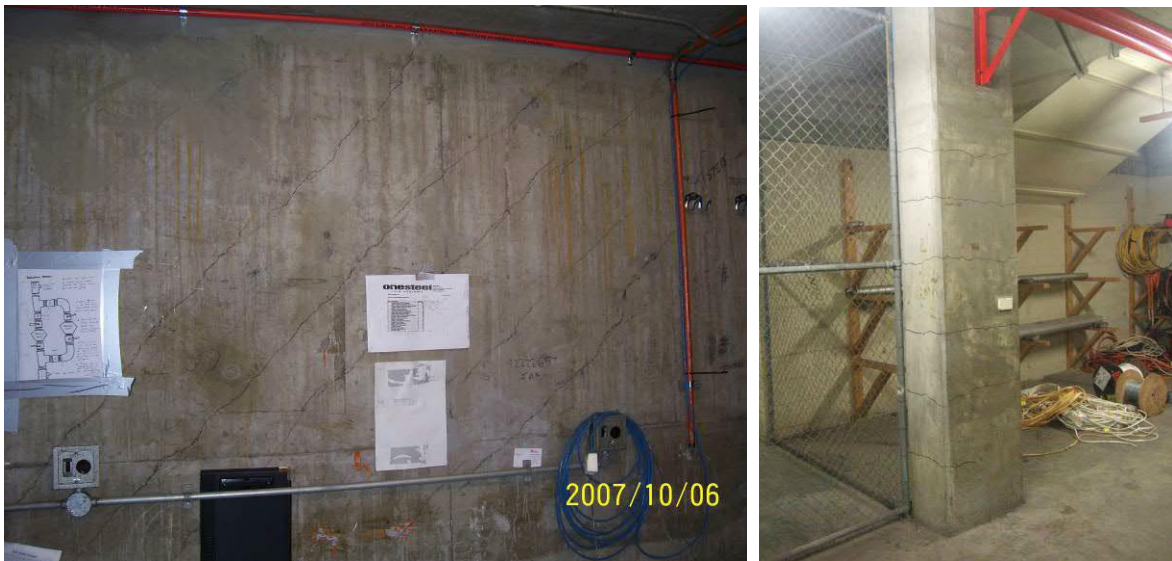
Figure 3 – Highly stressed wall (left) and column in tension (right) at upper levels (top) (source – Hyder Consulting)
