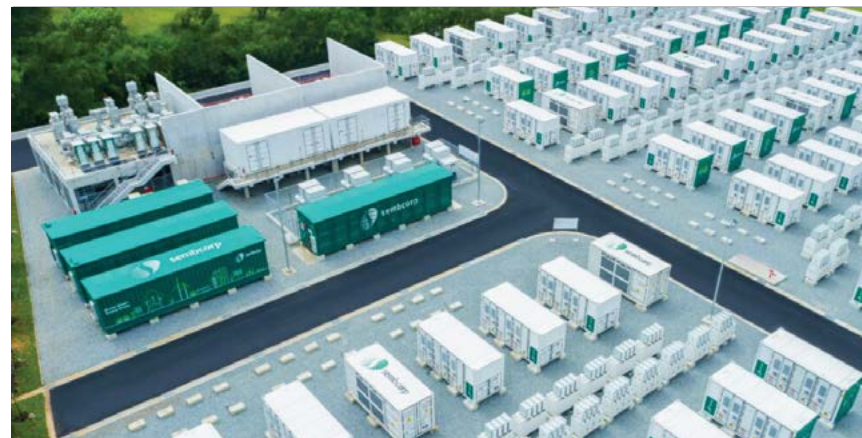
The 200MWh project on Jurong Island, Singapore. (Image: www.energy-storage.news © Sembcorp)
