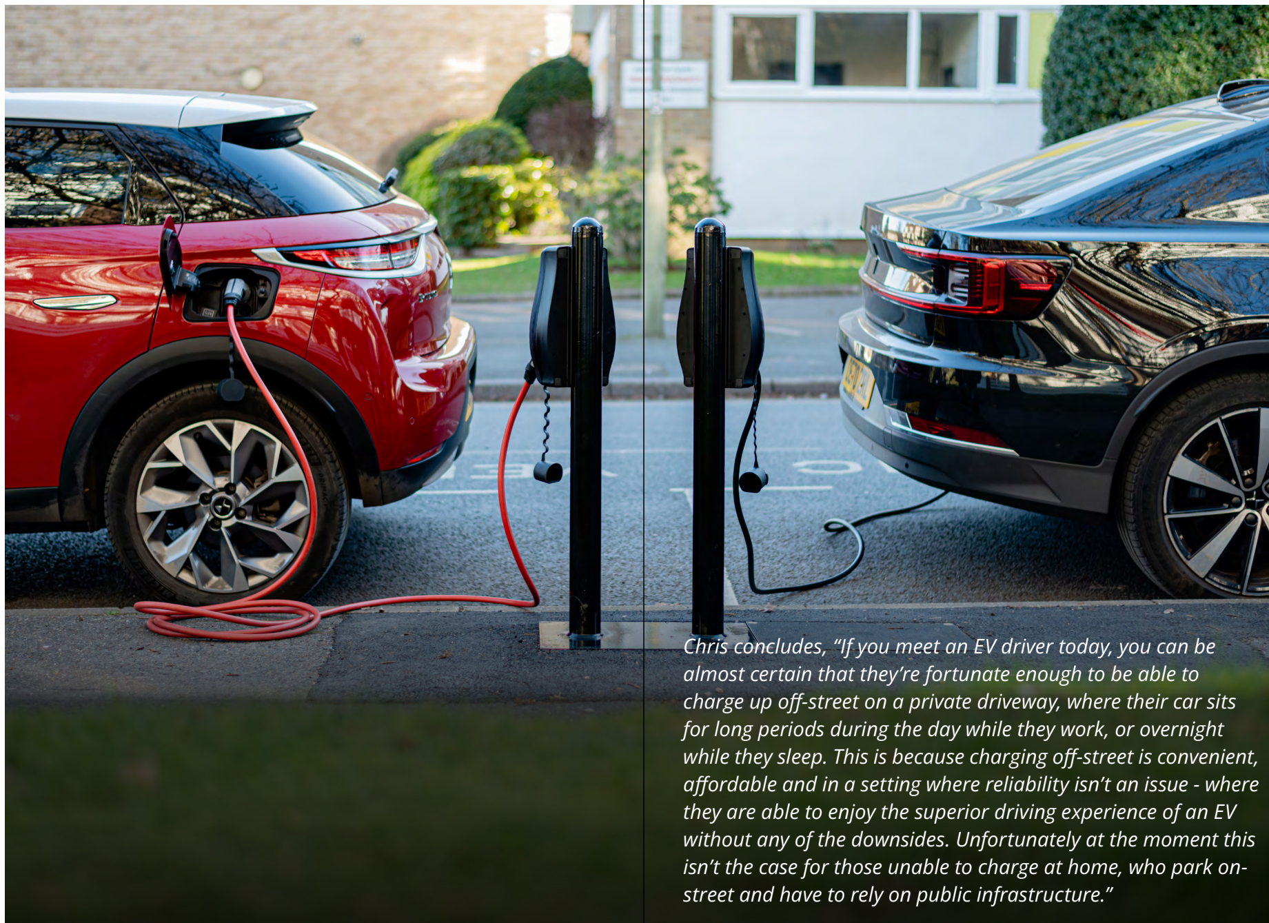
Connected Kerb charging stations. (Image: Connected Kerb)
