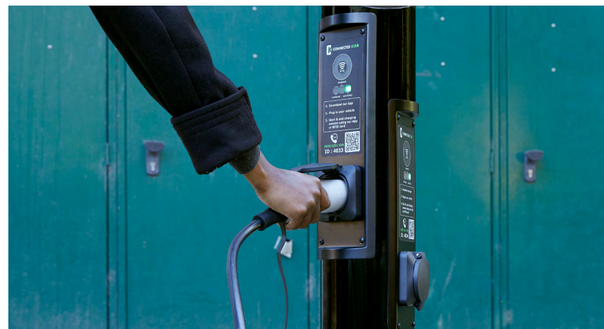
Connected Kerb charging station. (Image: Connected Kerb)
