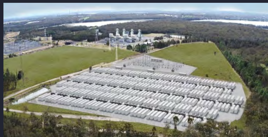
The new Waratah Super Battery will be capable of discharging up to 850MW/1680 MWh. (Image: Powin)
