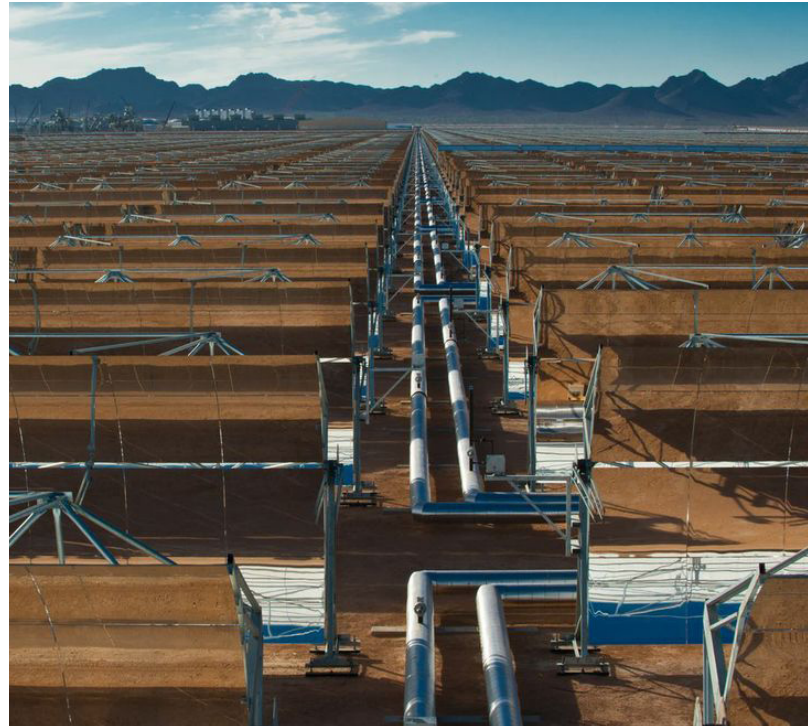
Abengoa Solar Solana power plant.
