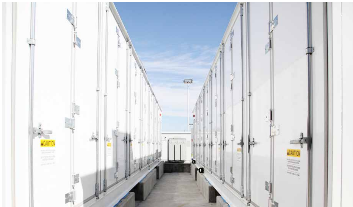
Photo courtesy of San Diego Gas & Electric
